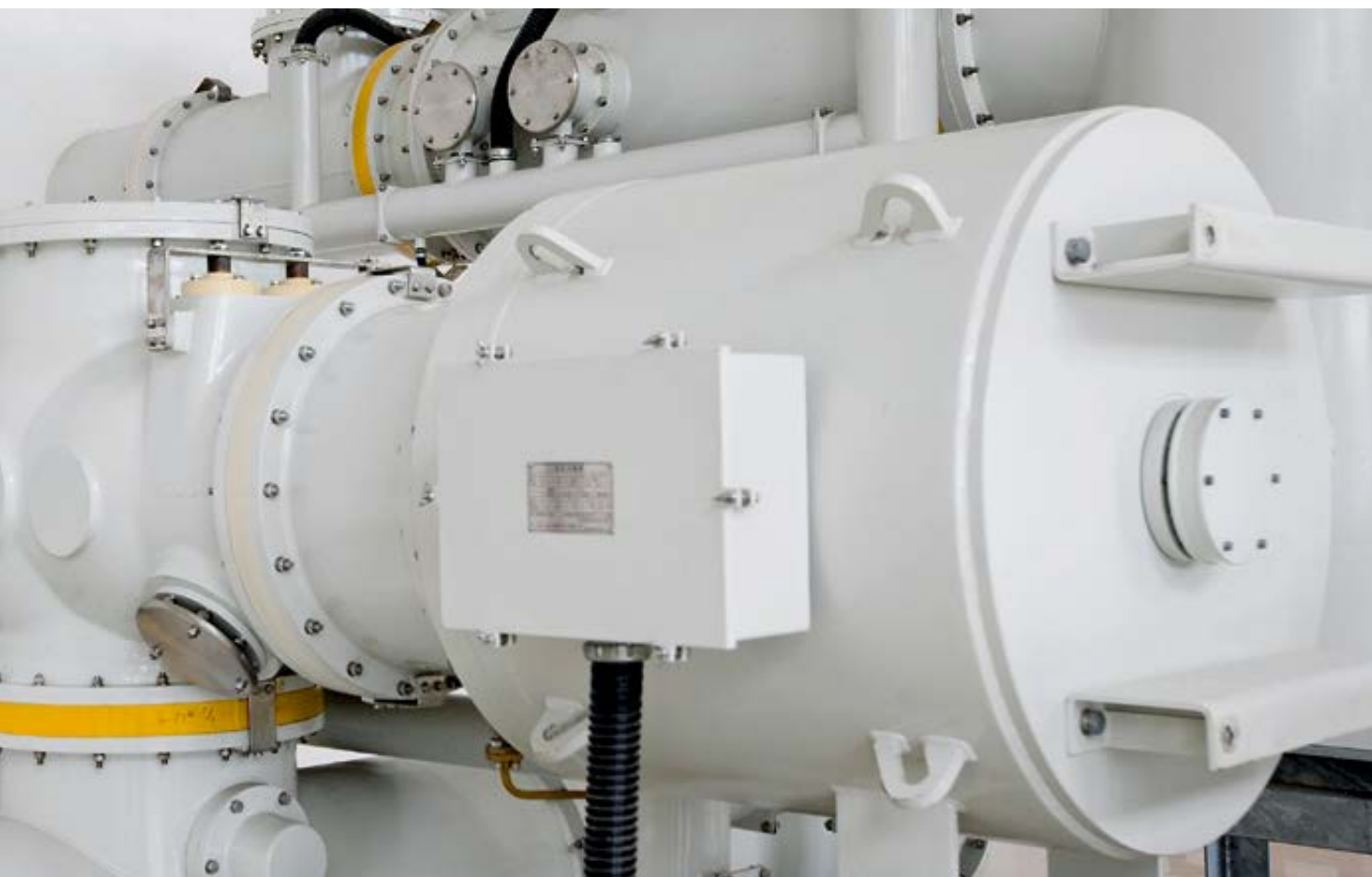
© Wind Power Works
